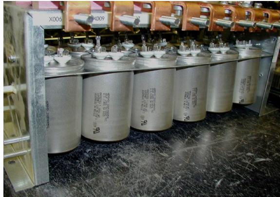
Figure 1 – UPS output AC capacitor bank
