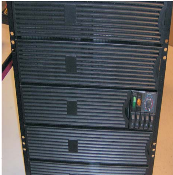
Figure 9 – Rack-mounted server simulator has adjustable heat and air flow settings
